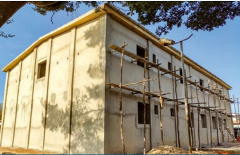
Through TRICE support, the new laboratory building should be finished by the end of 2021, Côte d'Ivoire
